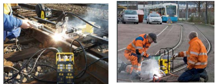
Fig.5 a) Railtrac - automated welding solutions for the repair of rail track components - ESAB; 5 b) Tramtrac™ II – for the repair of embedded city tramway rails - ESAB [3].
