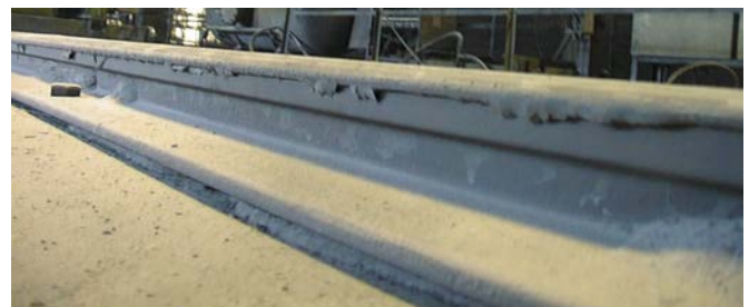
Fig. 2. The wear of the driveway with the flowing phenomenon.
